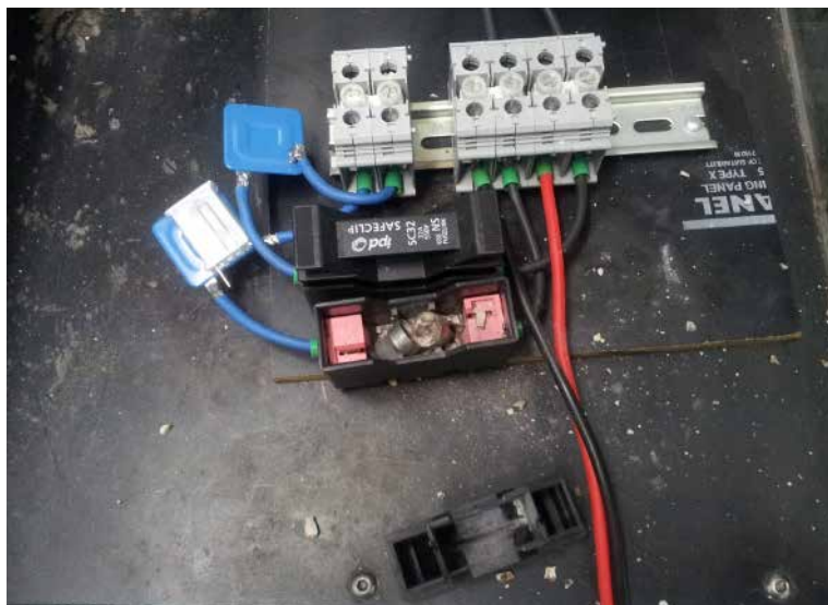
Figure A7. 32A Fuse Destroyed After One 22kA Impulse
